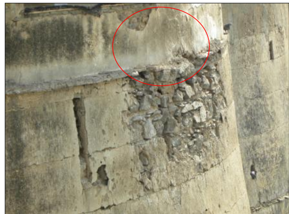
61. Lachmangarh Fort, Rajasthan: Piling of plaster on fortification due to exposure to open weather
