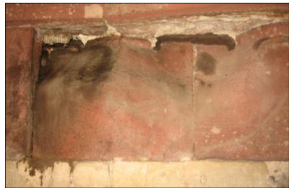
57. Muhammad Shah's Tomb, Lodi Garden, Delhi: Damages in sandstone ashlar blocks due to rusted iron member
