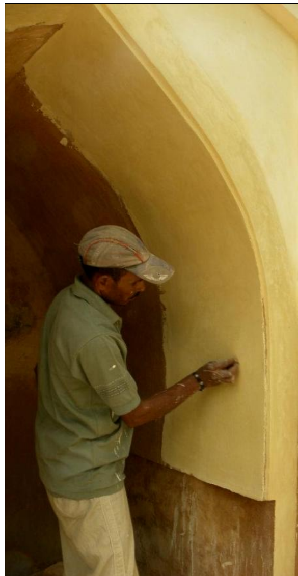
63. Mosque of Darwesh Shah, New Delhi: Finishing and smoothening of plastered surface by application of lime punning over it
